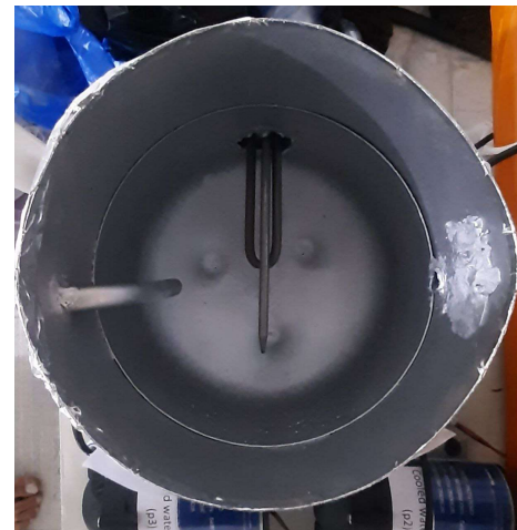
c. heating system
